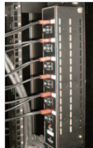
Figure 7. A zero-U power distribution unit provides power to 48V input loads.
